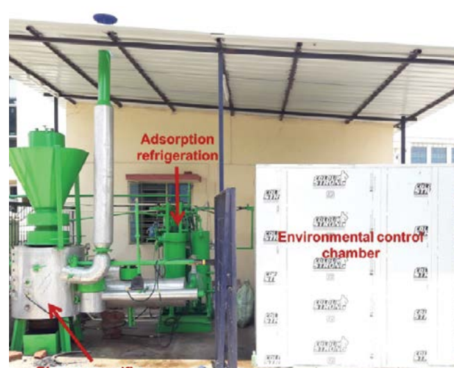
Biomass Gasification powered Adsorption Refrigeration System
